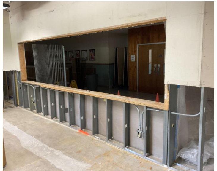
Renovation of the secure entry and reception area at Central MS is underway!
