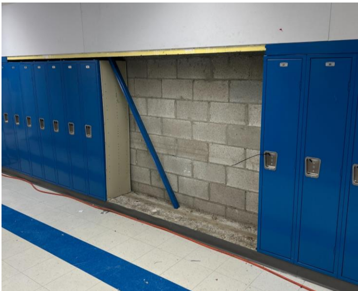
Lincoln ES lockers were moved in preparation for the new doorway into the special education classroom.
